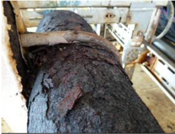
Figure 21: Picture of close up of pipe by pipe support shown in the picture above. Rust Building ca.10mm
