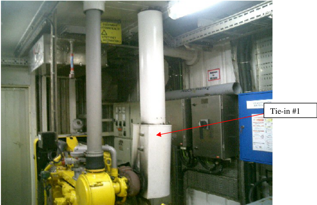
Figure 16: Tie in point 1 above bellows (inside insulation)
