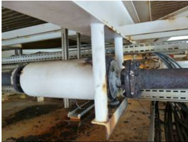
Figure 19: Picture of "muffler", this is extremely corroded with more holes. Some have tried patches as the picture shows
