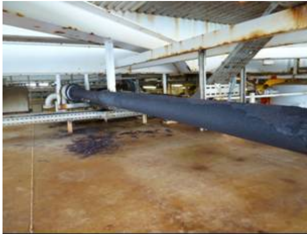
Figure 18: Overview picture of the pipe on the roof of the room for emergency generator
