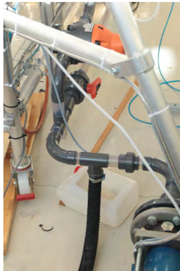
FIGURE 3.6: Open/Close valve for directing the flow into the circulation path
