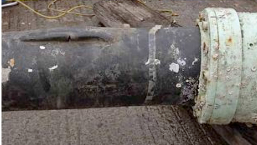
Figure 6 - Rupture of external sheath due to leak in end fitting [11].
