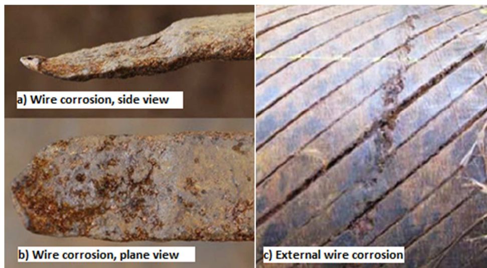
Figure 14 - Corroded tensile armour wires due to breach of outer sheath [1].
