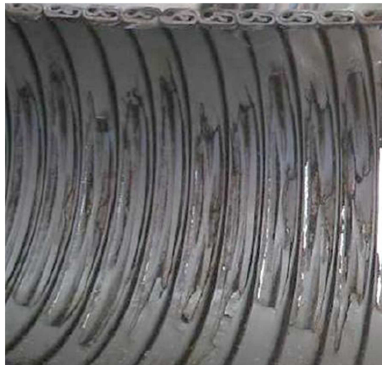
Figure 13 - Internal erosion of carcass [1].
