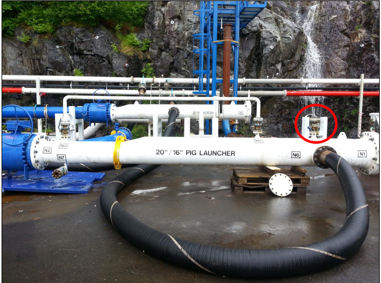
Figure 12 Pig-launcher and pig-receiver mounted on the test loop
