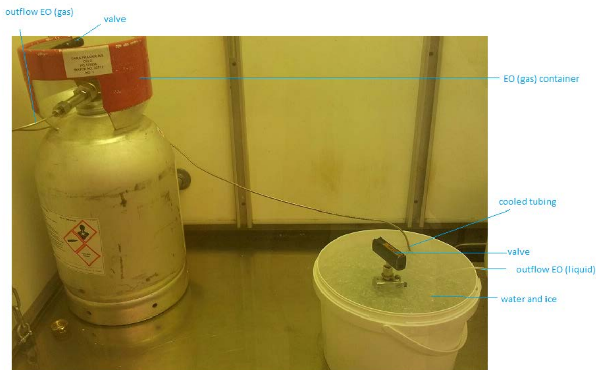
Figure 16: The cooling system of EO (gas to liquid)
