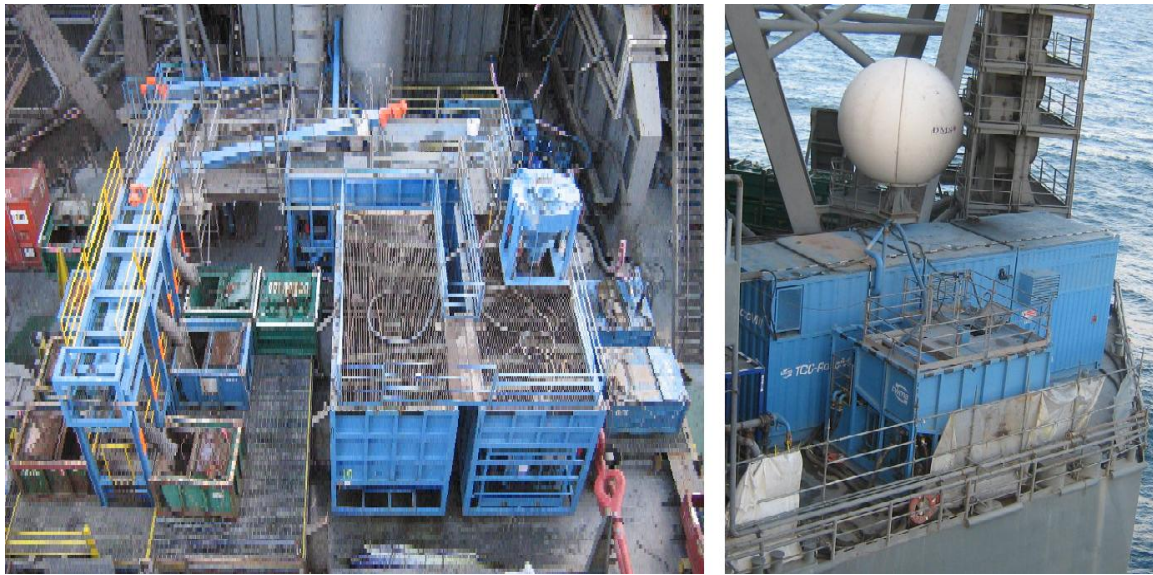
Figure 11: Rowan Gorilla 5: Skip station, buffer tanks and TCC unit installed (Gregoire, 2013)
