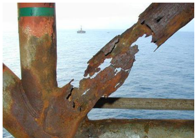
Figure 5.1.1 corroded support structure on an offshore installation [18]
