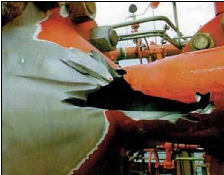
Figure 1: An eroded wellhead piping [9]
