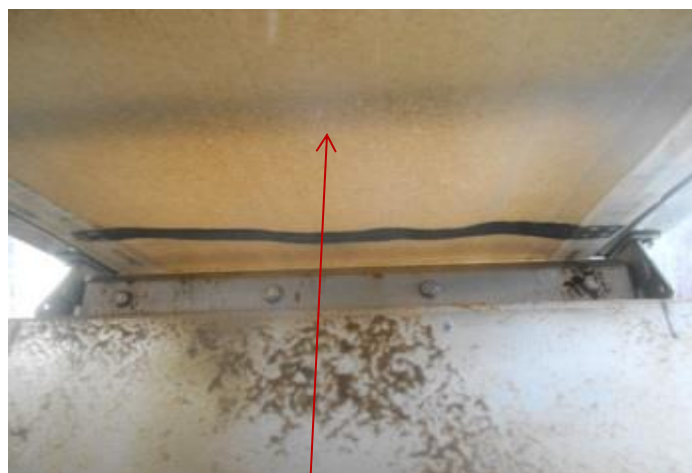
Scraper unable to clean mesh sieve completely
