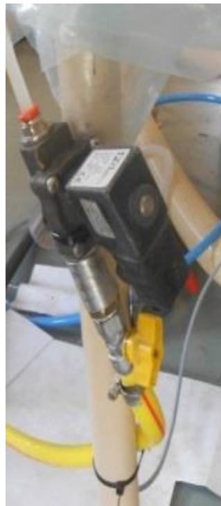
SF500 wash water solenoid valve
