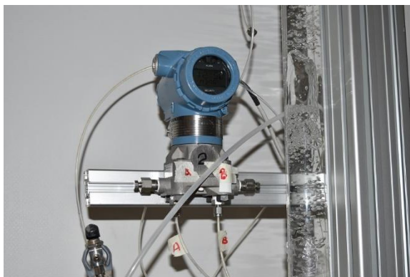
Figure 44- Rosemount 3051C pressure gauge differential pressure measurer
