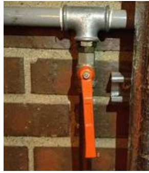
Figure 45- Open position of Valve 1
