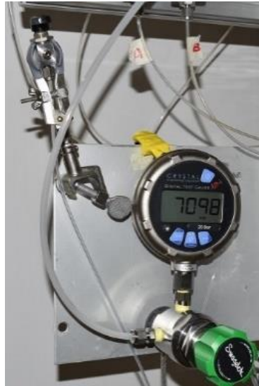
Figure 42- Switch directing gas towards open atmosphere; gas regulator, and inlet pressure Crystal Digital test; Gauge XP2i manometer
