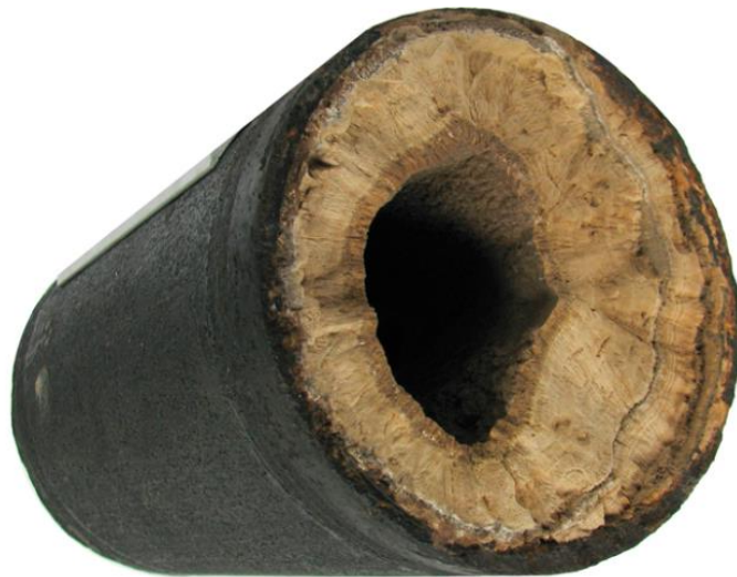
Figure 2-1: Scale built up in plumbing pipes [10]
