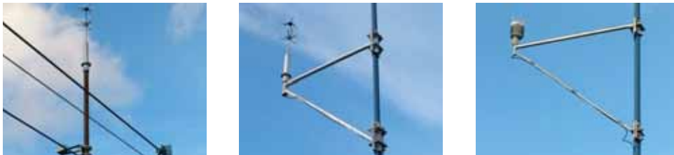
Figure 3.5 Sonic anemometer on H-24 (left), on H-18 (middle) and weather station on H-10 (right) installed 6 m above the West side of the bridge deck.
