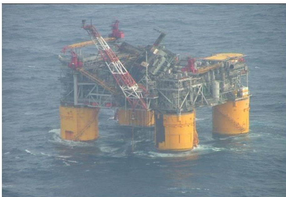
Figure 2.1 Mars platform was damaged in 2005 (Ove T. Gudmestad, 2006)
