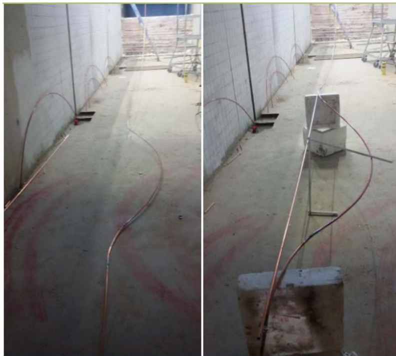
Figure 6-15: Pipe Rotation with a 2m R.C of 0.40% Residual Strain and 2-spring Pipeline Bottom Condition
