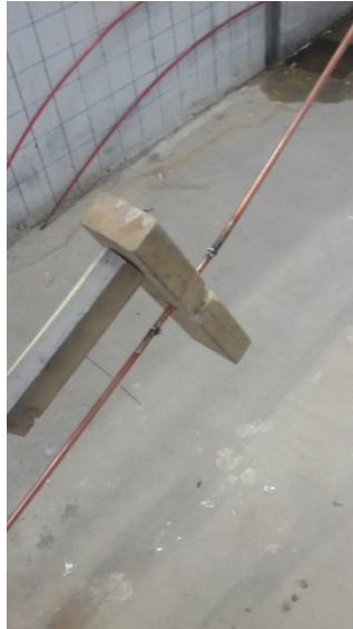
Figure 4-15: Inline Structure Connected to the Pipeline
