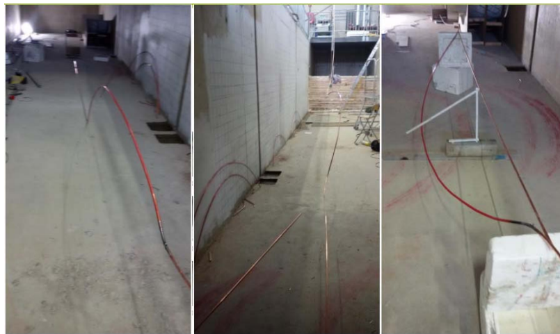
Figure 6-17: Pipe Rotation with a 3m R.C of 0.35% Residual Strain and 2-spring Pipeline Bottom Condition
