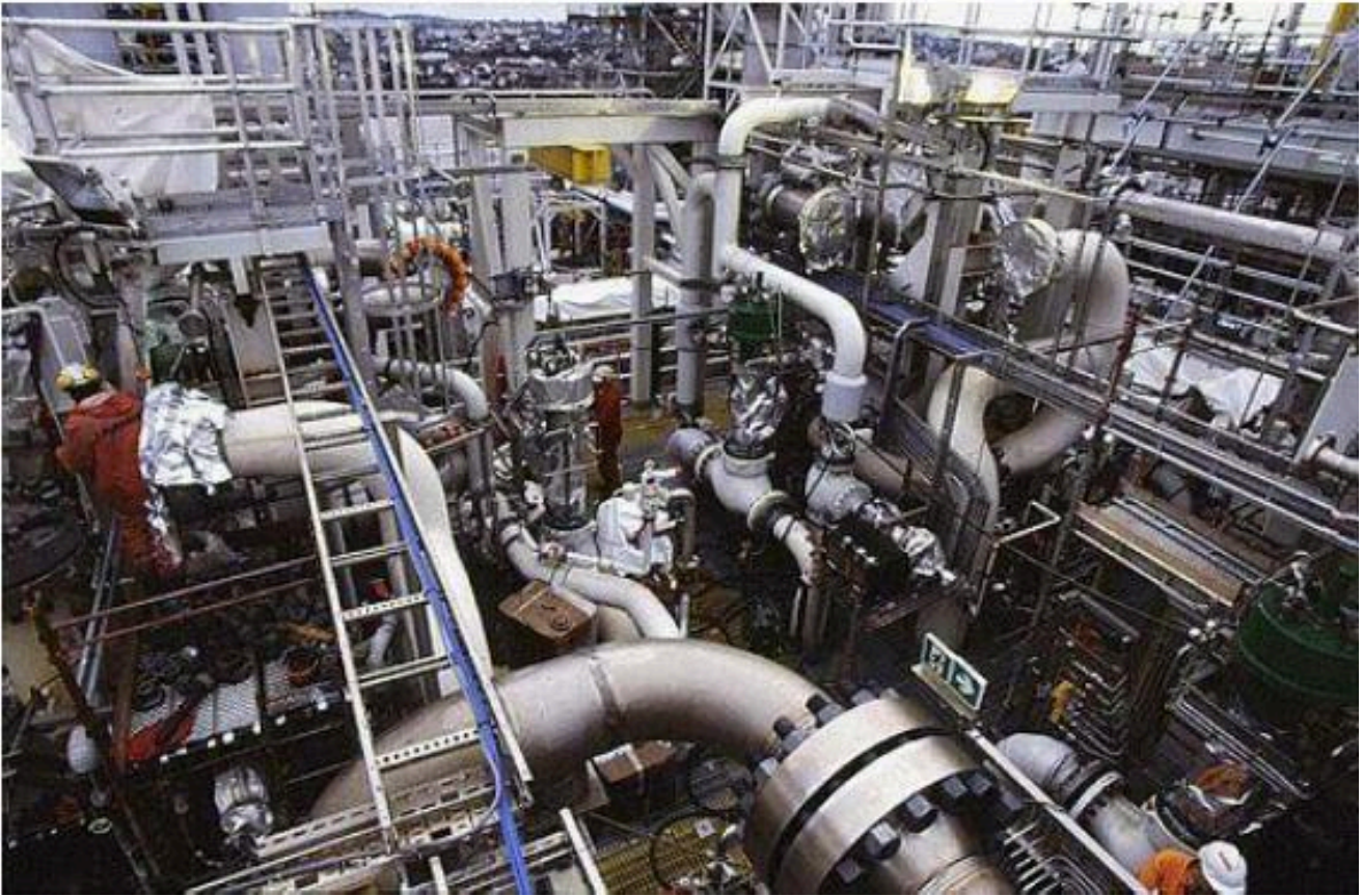
Figure 8: Adequate space must be provided around machinery, tanks, vessels, and pipe-headers. (Odland, 2015)
