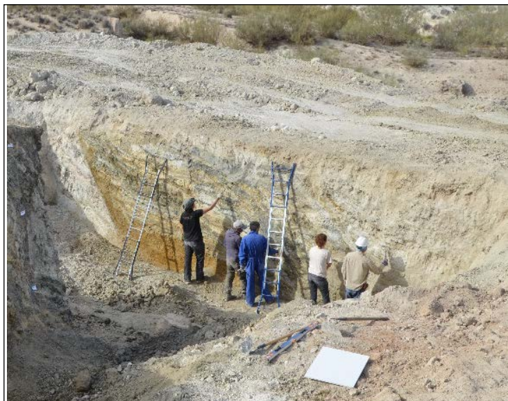
Figure 13: The team working together to remove the debris from the fresh surface using hand tools.
