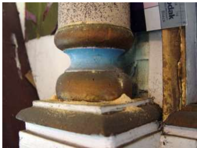
Picture 19 Most of the wood worm holes were found at the columns.
