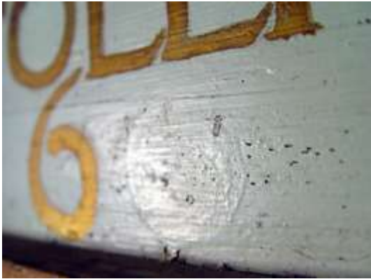
Picture 22 The original paint is marking off through the over paint in the glazing light.
