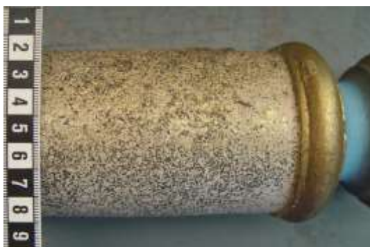
Picture 20 Detail of a column secondary paint: The columns are painted in light pink, decorated with bronze particles.
