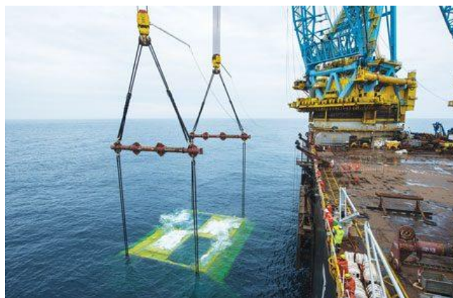
Figure 2.8: installation of the Åsgard subsea compressor manifold station in summer of 2003 from the Saipem 7000. Courtesy of Statoil. (Davies & Ramberg, 2016)
