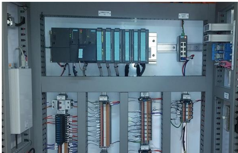
Figure 28: Siemens Sematic S7 400 – PLC. (Wagtec.com, 2018)
