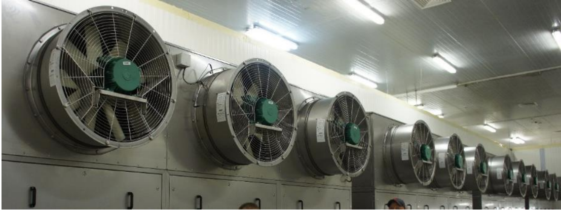
Figure 32: Chiller air circulation fans (Gate Gourmet)
