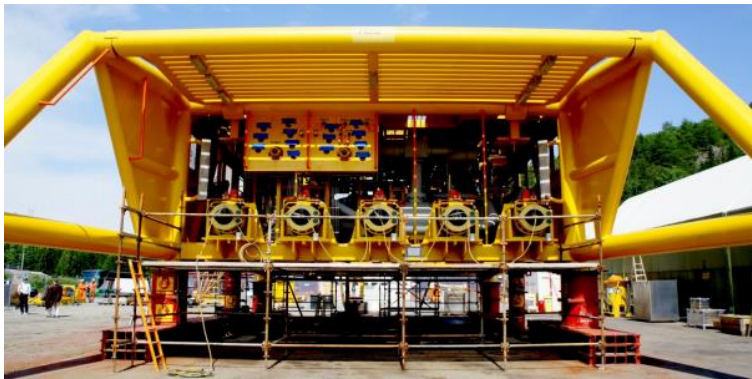
Figure 12 – Kirinskoye Subsea Manifold [17]
