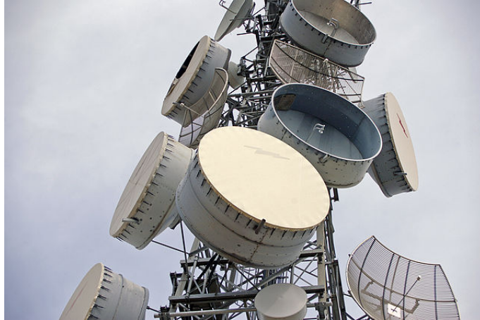
Figure 2.2: Photograph of parabolic dish antennas placed on an antenna tower [2].
