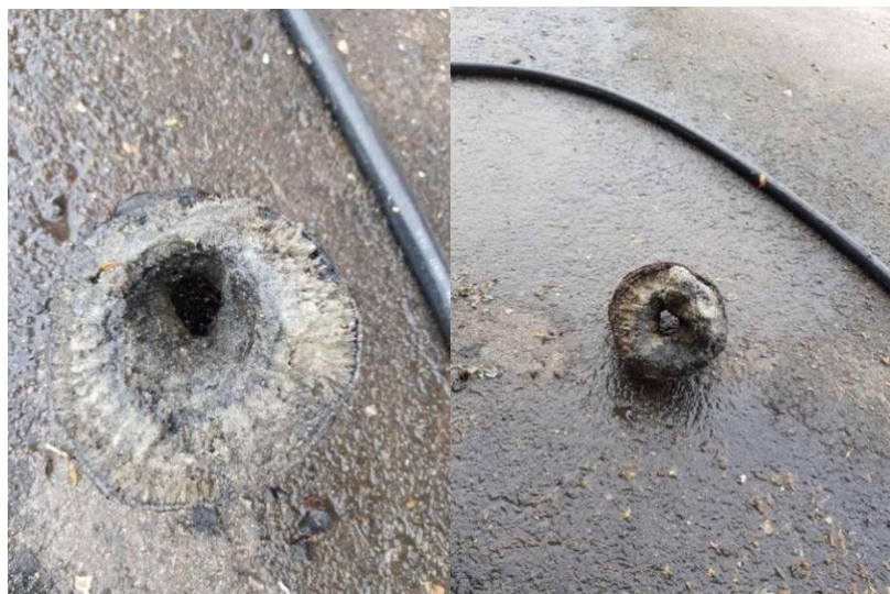
Figure 4.25. Struvite formation in piping downstream centrifuges at SNJ.
