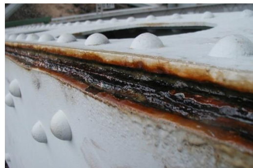
Figure 3: Example of Crevice Corrosion (Steelfab, 2017a)
