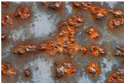
Figure 5: Example of Intergranular Corrosion (Steelfab, 2017c)
