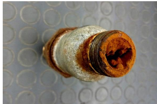
Figure 6: Example of Galvanic Corrosion(Steelfab, 2017b)
