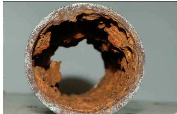
Figure 9: Example of Microbial Influenced Corrosion (Tanks, 2017)
