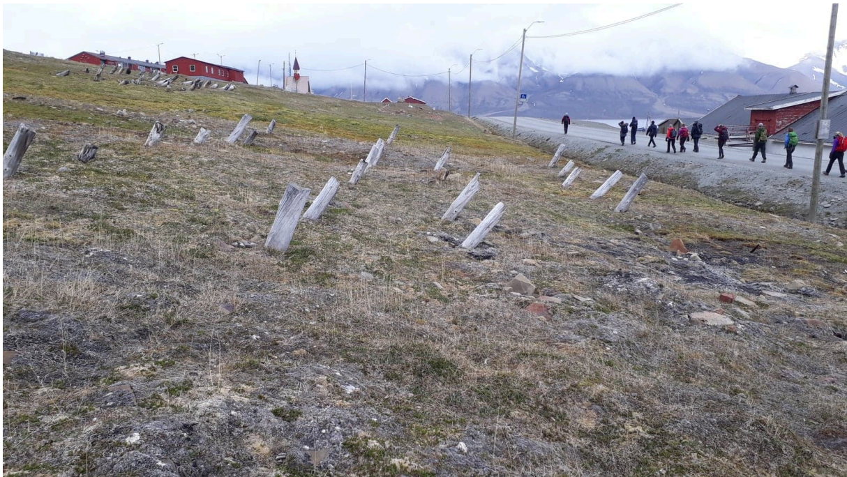
Figure 5: Example of how the active layer affects structures on Svalbard. Here you can see remaining piles that have been tilted due to downward movement of the active layer. Photo: Viktor Gydemo, June 2018.
