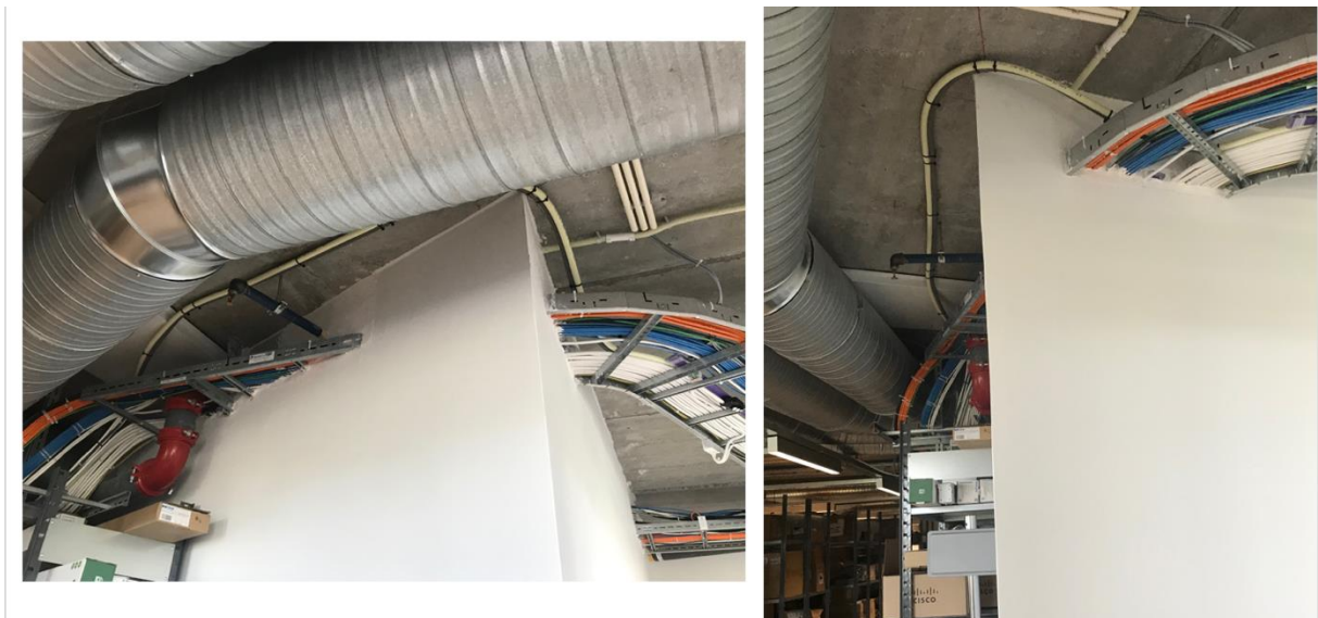
FIGURE 31 A PICTURE OF THE CURRENT SITUATION (SEEN FROM ONE SIDE), (ATEA, PERSONAL COMMUNICATION, JUNE 2019)
