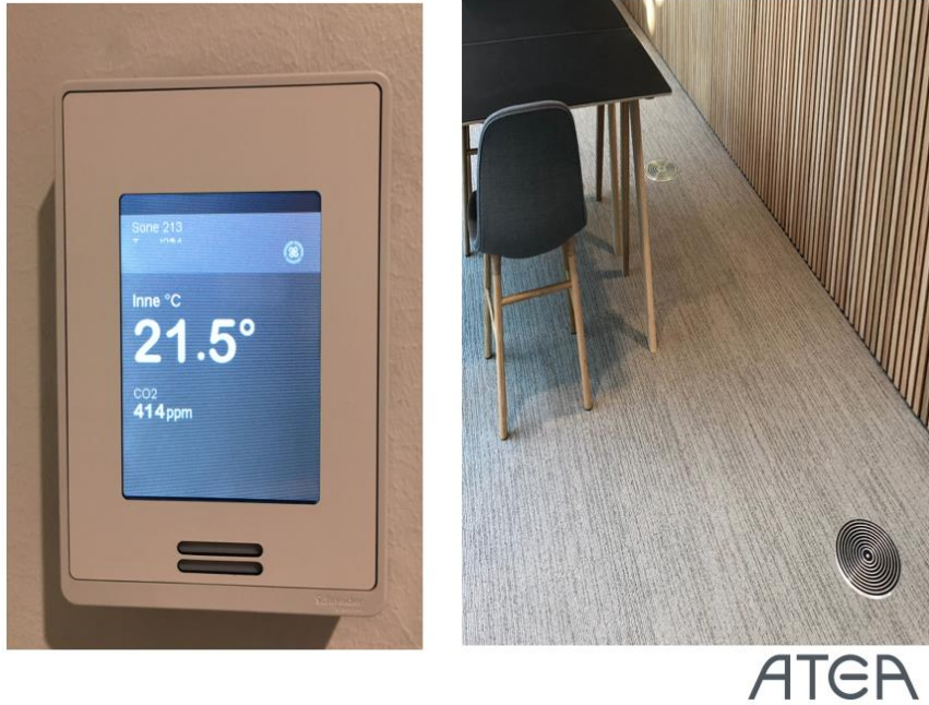
FIGURE 27 A PICTYRE OF THE SCREEN OUTSIDE ONE MEETING ROOM, SHOWING TEMPRATURE AND CO2 LEVEL, (ATEA, PERSONAL COMMUNICATION, MAY 2019)
