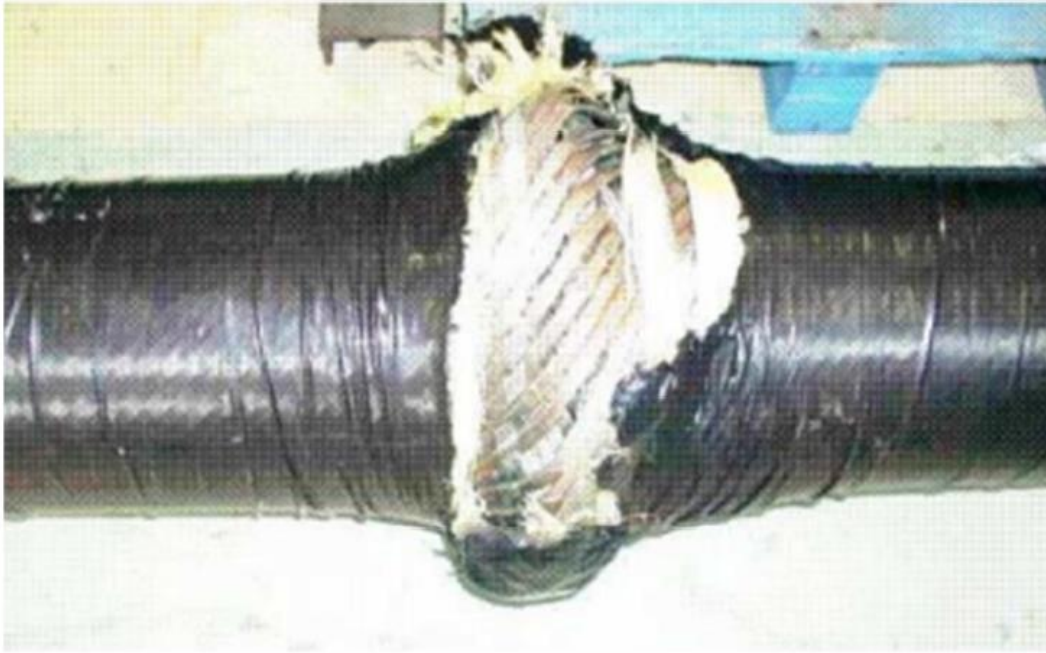
Figure 54 Shows an example of radial buckling (bird-caging)[54].
