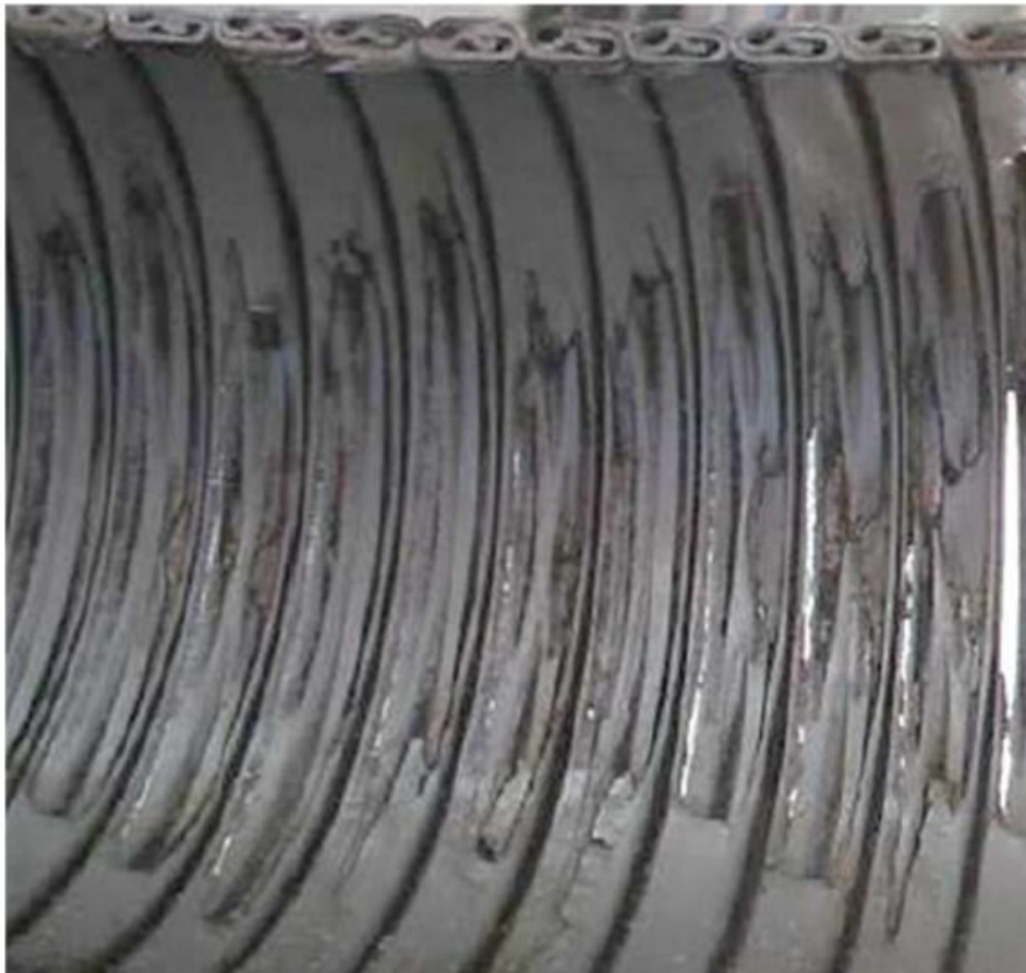
Figure 56 Shows internal erosion of carcass[19]
