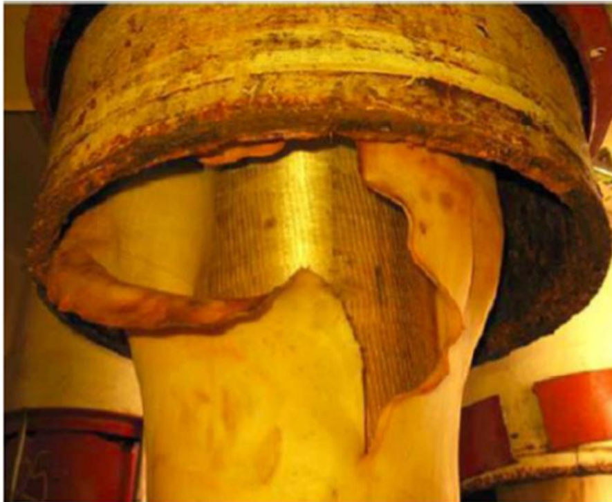
Figure 51 Rupture of the external sheath due to blocked vent tubes[19].
