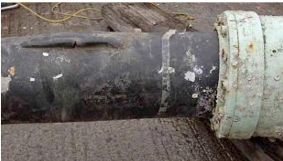
Figure 50 Rupture of external sheath due to leak in end fitting [51].
