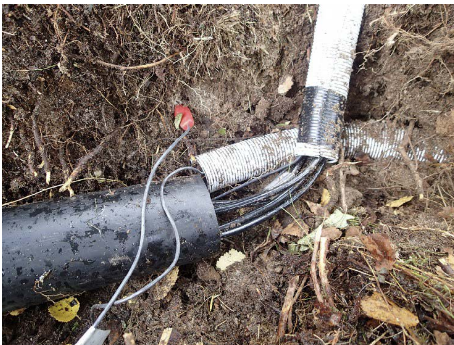
Figure 33: Location of reference probe, S of the BioForsk datalogger cabinet. The root zone is clearly seen. Photo: MVH Consult.
