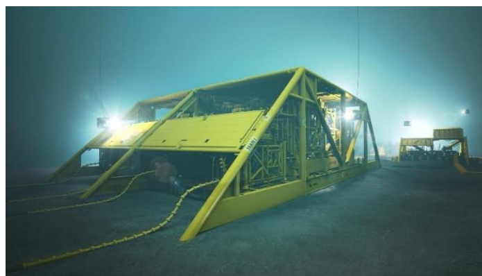
Figure 1-4 Subsea template on seabed at Åsgard field [Source: Equinor].
