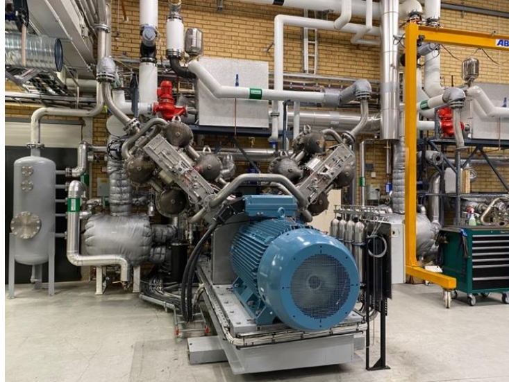
Figure 2: Illustration of a functional HighLift heat pump at Astra Zeneca's R&D facility in Gothenburg.
