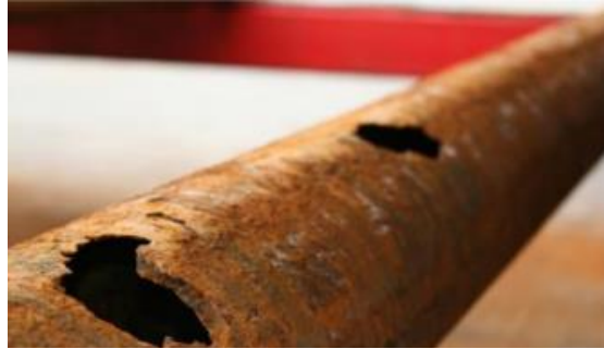
Figure 2-5: Corroded production tubing due to incompatibility between fluid and tubing.[13]
