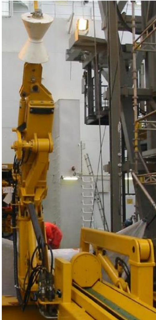
Figure 5-29: Tail in arm used to guide the pipes during pipe retrieval and deployment. [64]
