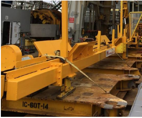
Figure 5-5: Catwalk machine installed on Island Valiant [31]
