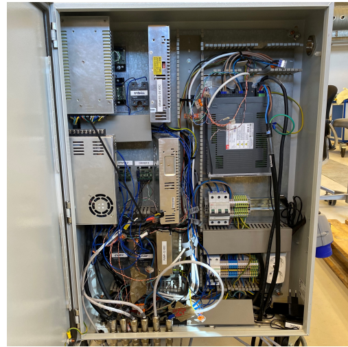
(b) Electric cabinet
