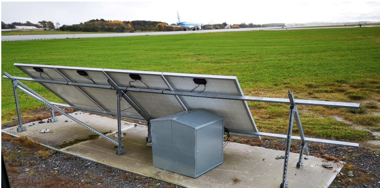
Figure 27: Image showing ground conditions of the green open space at Stavanger Airport with a solar PV panel in place for test purposes. (self-captured image during field visit)
