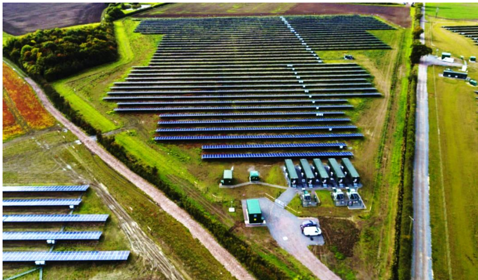
Figure 22: 10 MW Clayhill solar PV farm, UK, with 6 MW utility-scale batteries (source:powermag)
