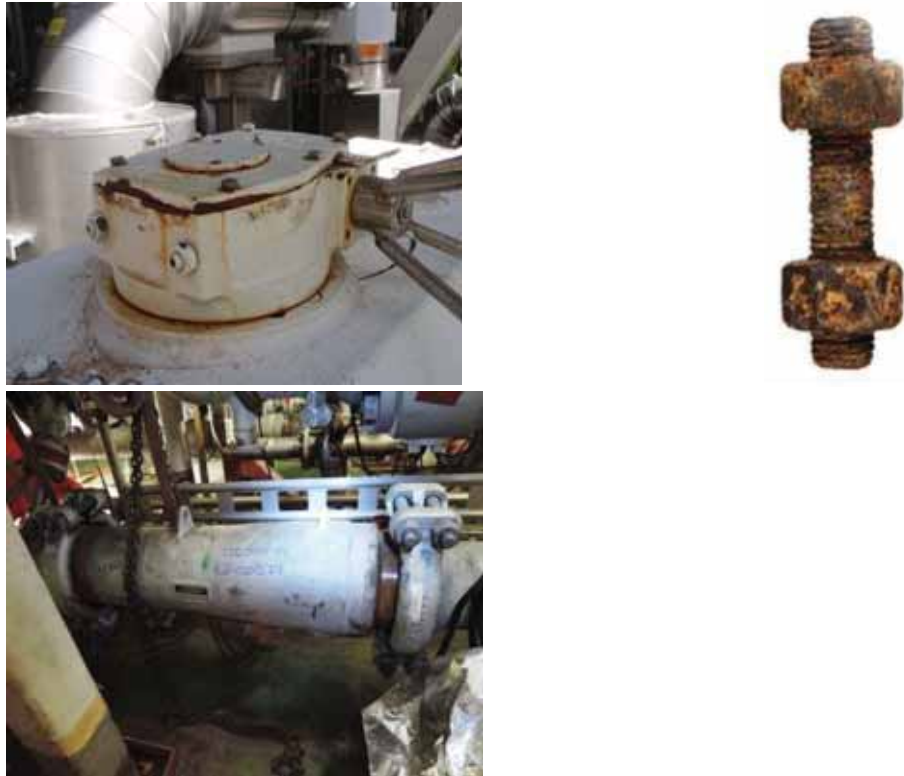
Figure 1: Corrosion of carbon steel valve / valve components
