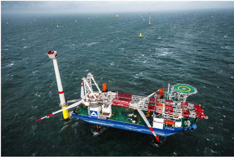
Figure A3-3 : Loading pre-assembled rotor and hubs and installation. (Press lease from global tech 1)
