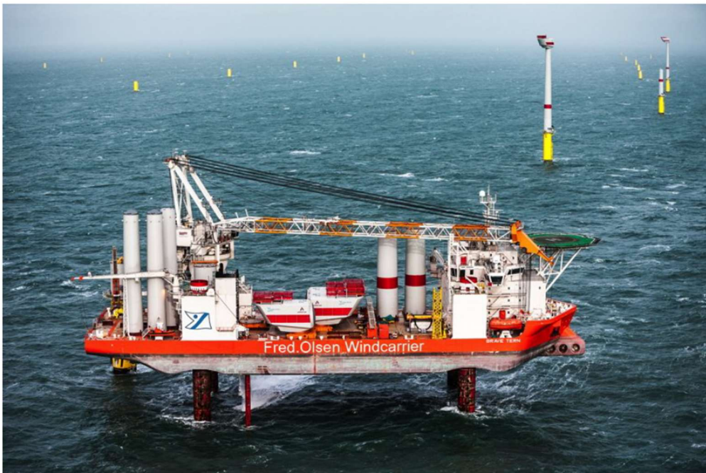
Figure A3-2: Loading and installing the tower and nacelle (Press lease from global tech 1)
