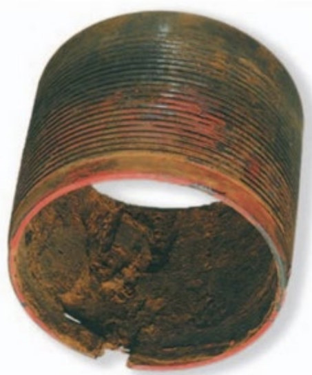
Figure 19 Carbon steel tubing (Bellarby, 2009)
