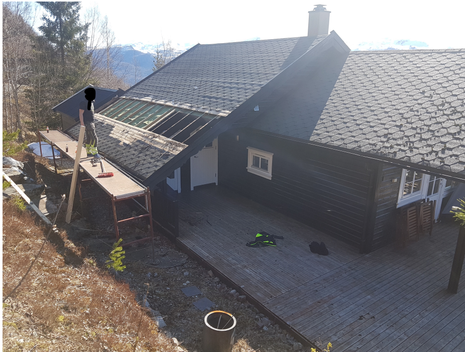
Figure 9: Moisture damage in the roof construction.
