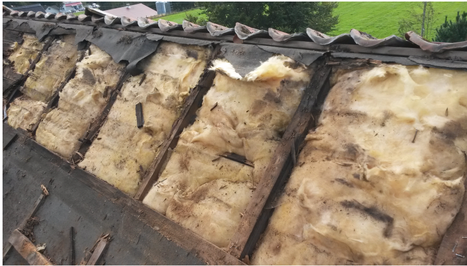
Figure 18: Signs of decaying material on the upper part of the roof beams.
