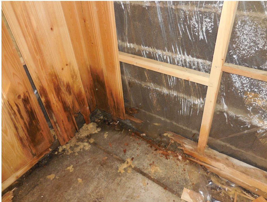
Figure 13: Moisture damage in bedroom.
