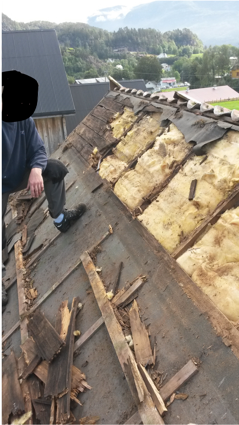
Figure 19: Significant decay along the entire length of the roof.
