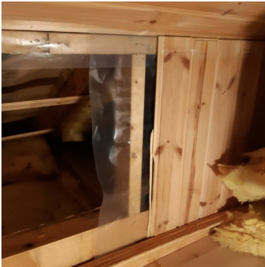
Figure 10: Knee wall located above bathroom and washing room. Visible is the lack of vapor barrier on the ceiling behind the knee wall.
