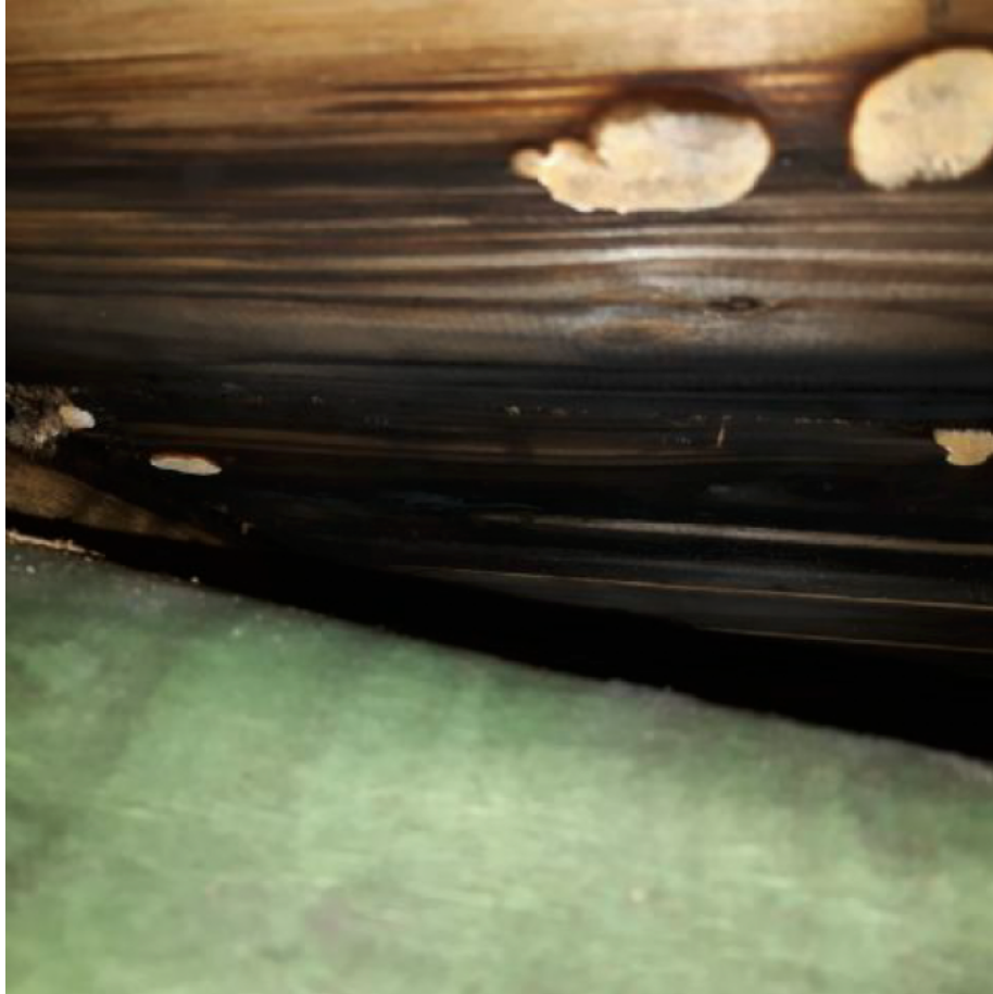
Figure 12: Visible fungus and mold on the inside of the roof sarking, as well as material starting to decay.
