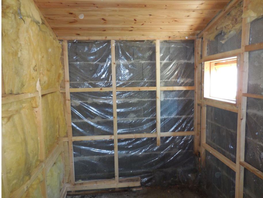
Figure 16: Overview of the room after opening the construction and removing moisture damaged parts of the walls.
