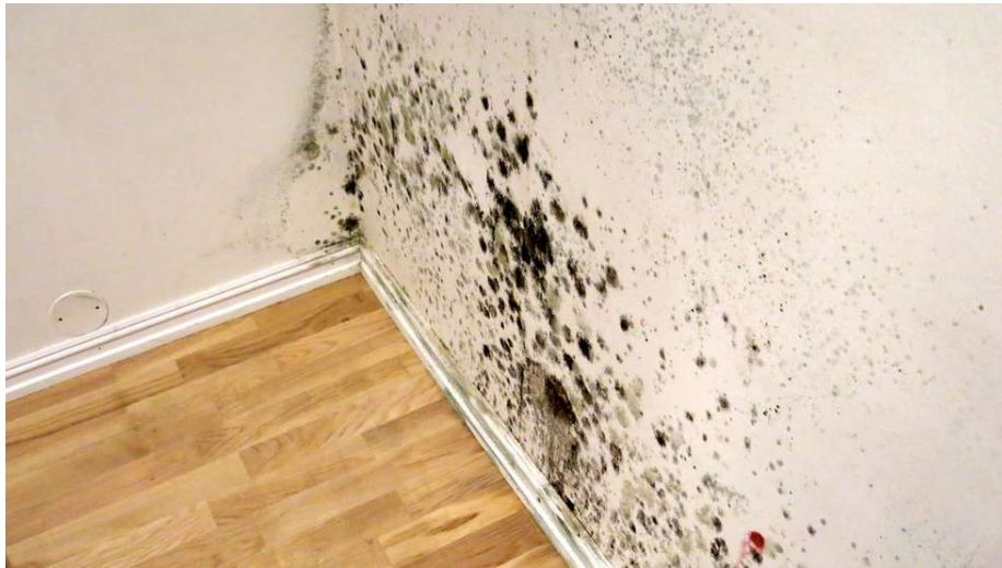
Figure 4: Mold and fungus appearing on interior wall found behind furniture [25].
