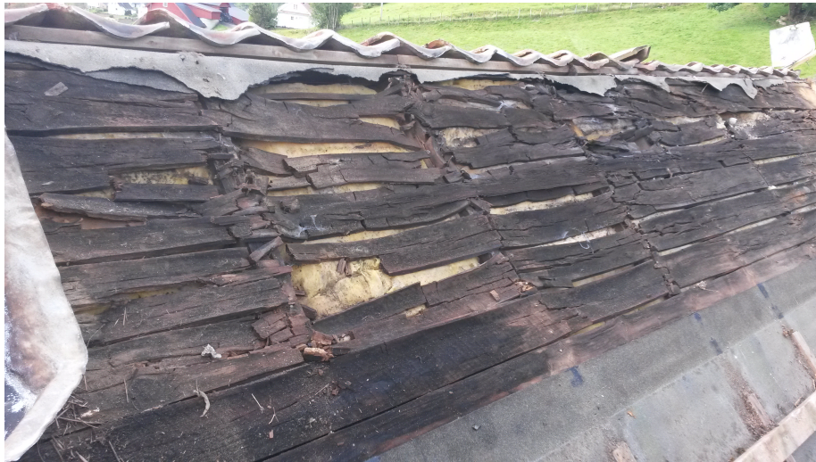
Figure 17: Moisture damage due to condensation in post-insulated roof.
