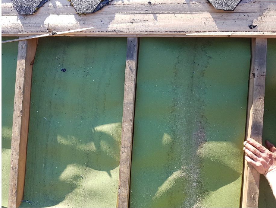
Figure 11: Visible signs of moisture and water on the wind barrier of the roof.
