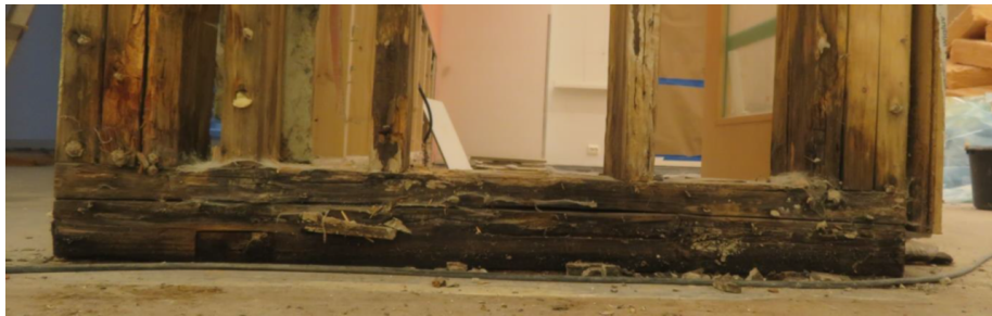
Figure 5: Decaying bottom sill caused by capillary suction [26].
