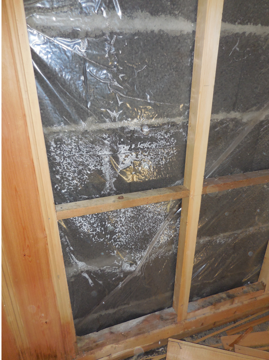
Figure 15: Visible condensation on the vapor barrier when removing the insulation.
