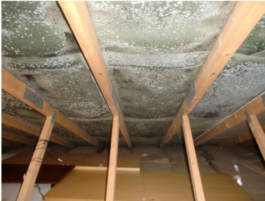
Figure 3: Mold on the inside of roof sarking in cold loft [24].
