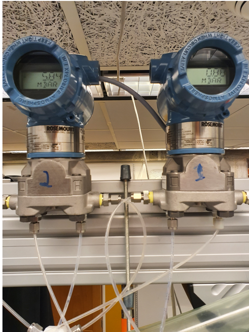
Figure B.10: Rosemount 3051 pressure transmitters. Nr 2 was faulty, Nr 1 measured pressure differences
