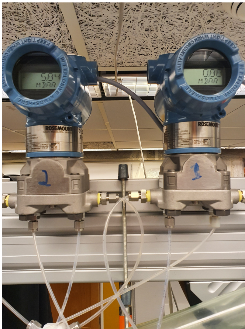
Figure B.10: Rosemount 3051 pressure transmitters. Nr 2 was faulty, Nr 1 measured pressure differences
