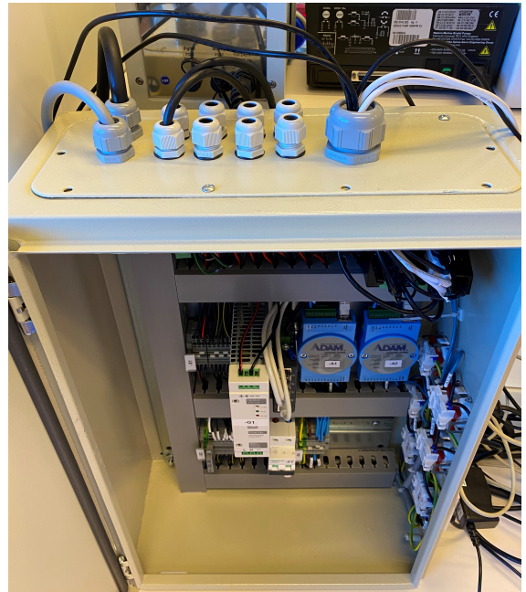
(b) Top side of the control cabinet with cable glands.
