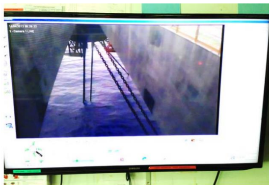
Figure 5.8. Monitor screen in control room for an FPSO [2]
