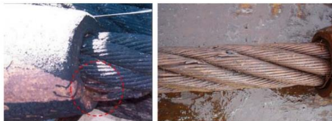
Figure 5.7. Broken wires at wire rope termination [32]
