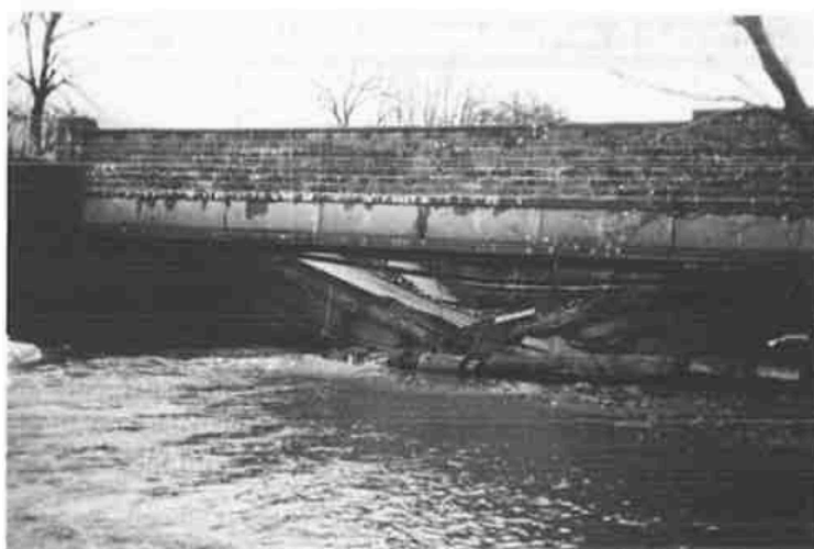
Figur 35: Ynys-y-Gwas etter kollaps [60, s. 40]
