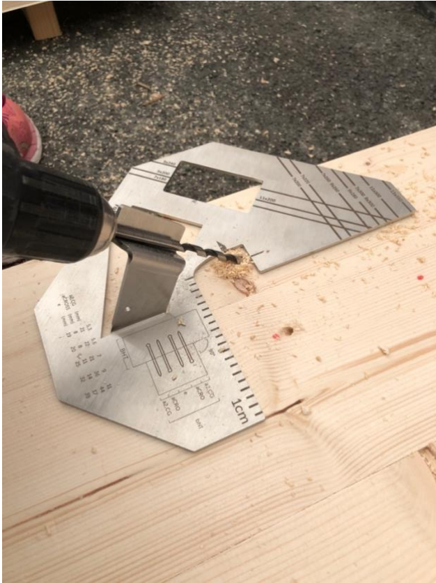
Figure 5-7 Pre-drill of a hole with a 6 mm wood drill bit by using the jig
