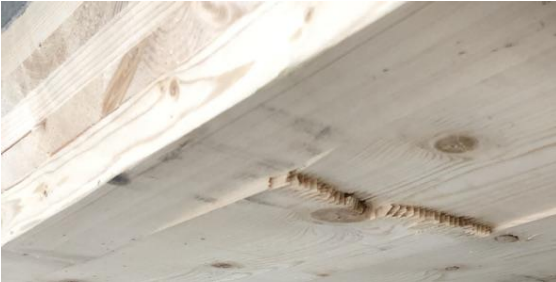
Figure 8-3 Finger joint and knot failure in the timber
