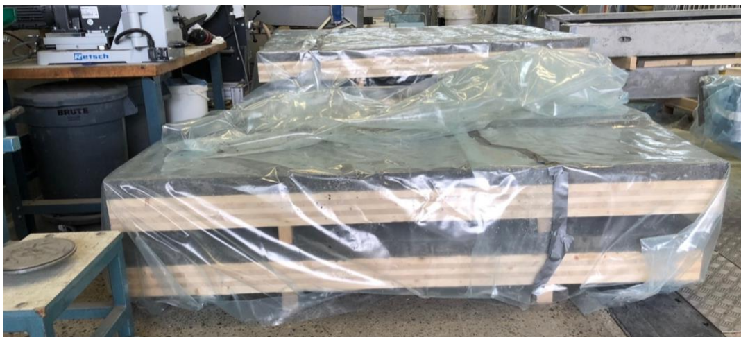
Figure 5-21 Curing of the CLT-concrete composite slabs using plastic covers after removing the formwork
