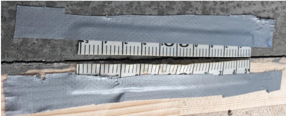
Figure 7-8 Movement in concrete and timber for Slab A4 at midspan
