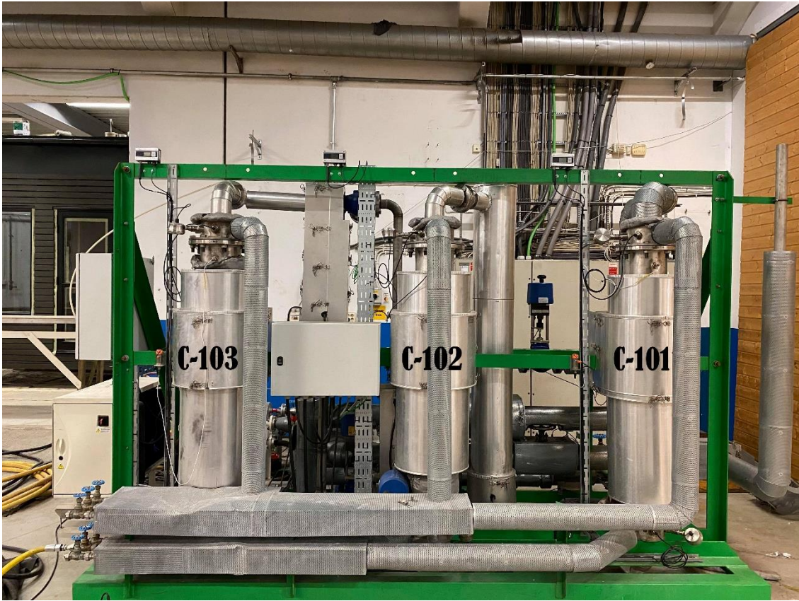
Figure 3.1: The front-side view of the Z8 test plant
