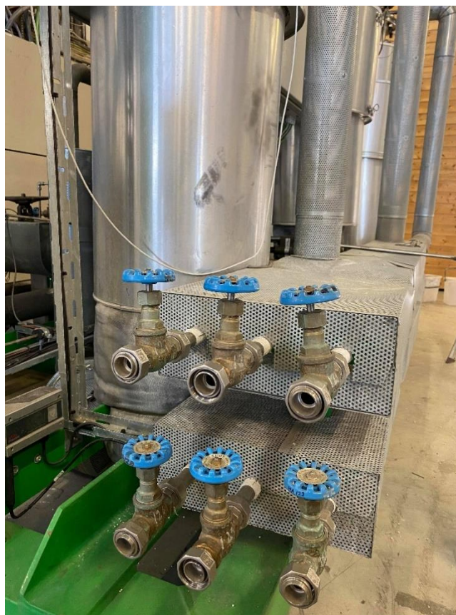
Figure 3.7: Bypass lines from adsorption columns
