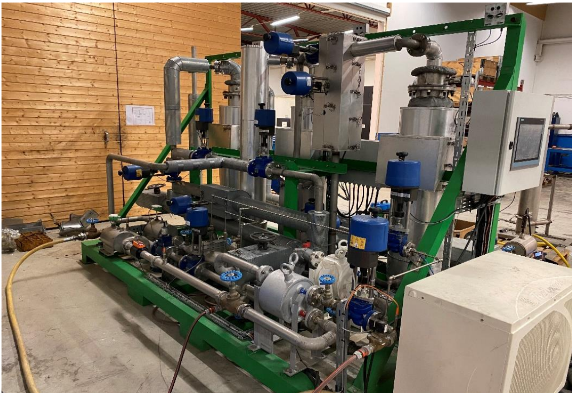
Figure 3.2: The back-side view of the Z8 test plant
