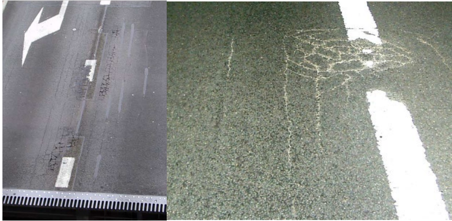
Figure 1. Indication of the presence of deck plate cracks [1].
