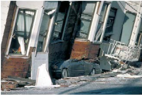
Figur 47 – Soft story collapse
