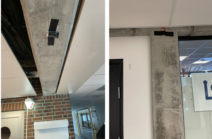
(a) ESP32 attached to the bottom of a vertical beam going across the ceiling (b) ESP32 attached to the side of a pillar
