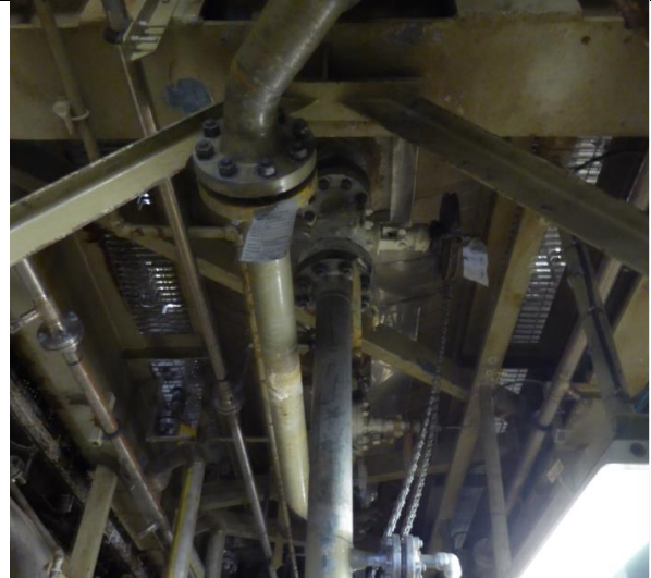
Picture 2. Separator insulated, picture taken from the bottom part. Lack of access due to supporting structure.
