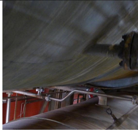
Picture 10. Separator not insulated, picture taken from the bottom part. Easy access from lower vessel.
