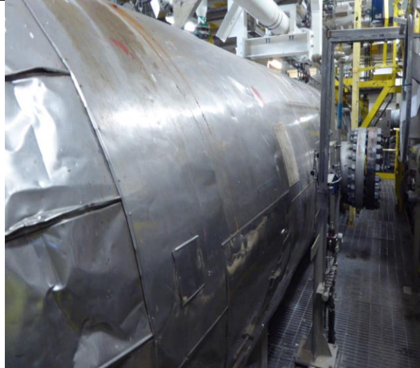
Picture 1. Separator insulated, picture taken from manhole side.
