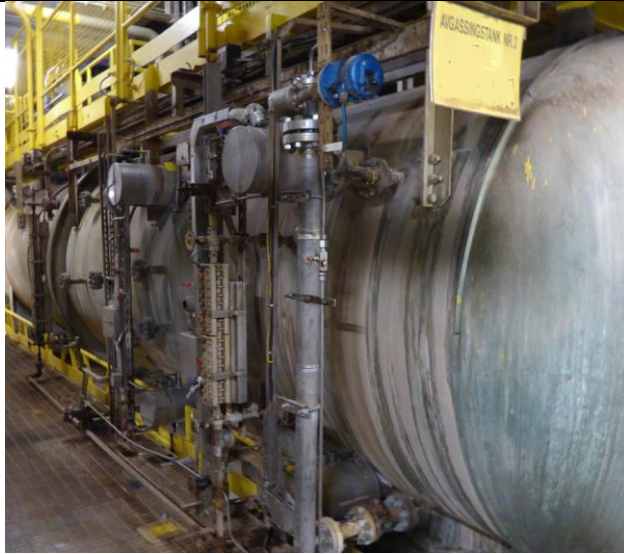
Picture 9. Separator not insulated, picture taken from manhole side.
