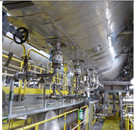
Picture 8. Separator insulated, picture taken from the bottom part. Easy access from deck.
