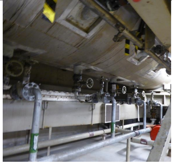
Picture 6. Separator insulated, picture taken from the bottom part. Easy access from floor.
