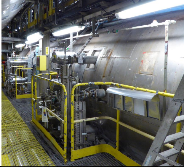
Picture 5. Separator insulated, picture taken from manhole side.
