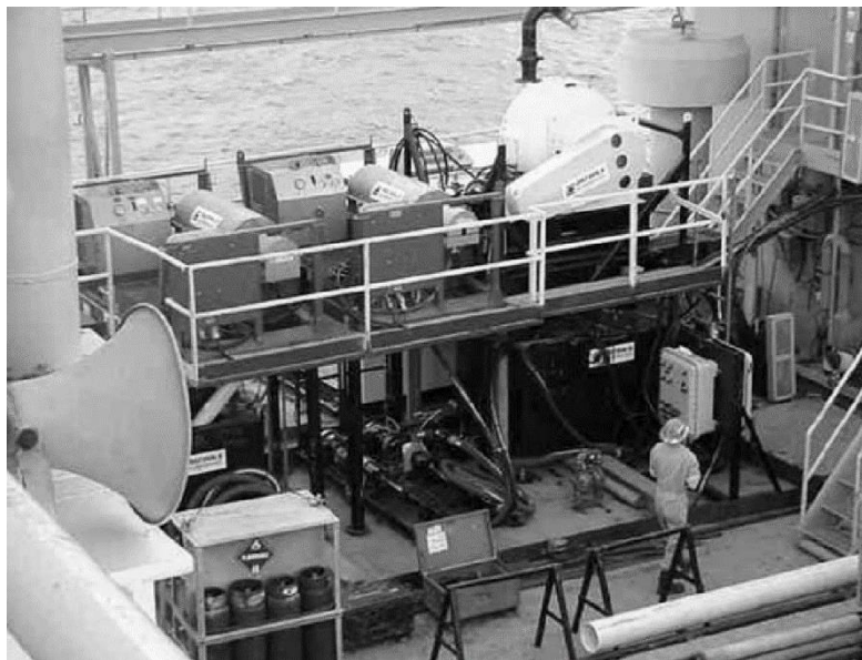
Figure 8: Horizontal cuttings dryer installation (American Society of Mechanical Engineers. Shale Shaker, 2005)
