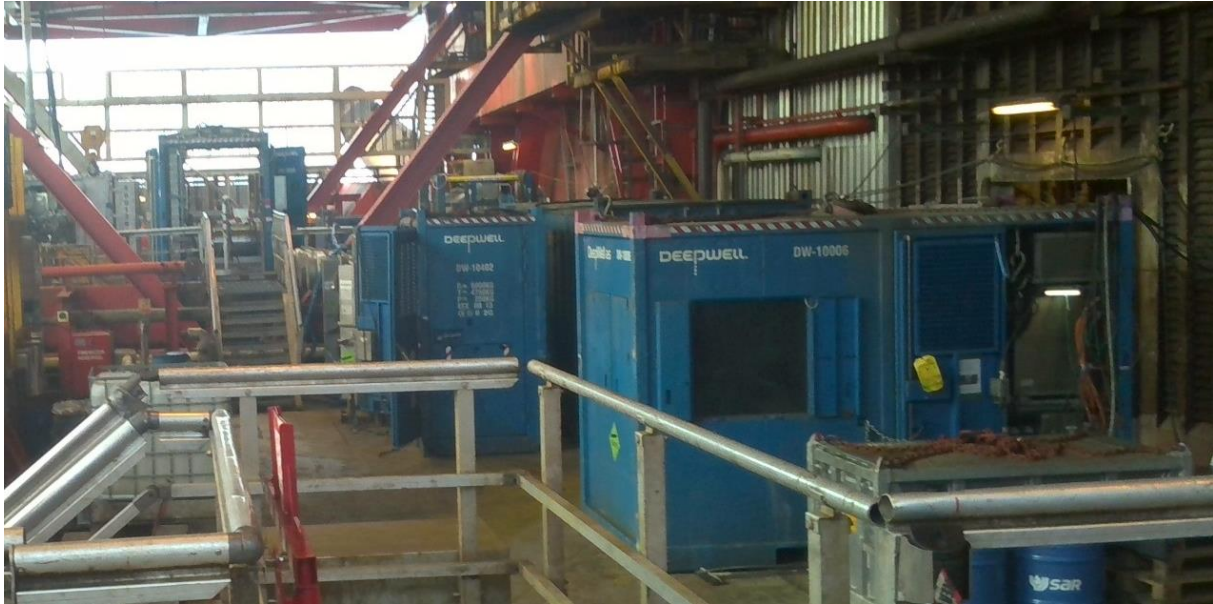
Figure 8: Winch control cabin, power pack and add on drum offshore
