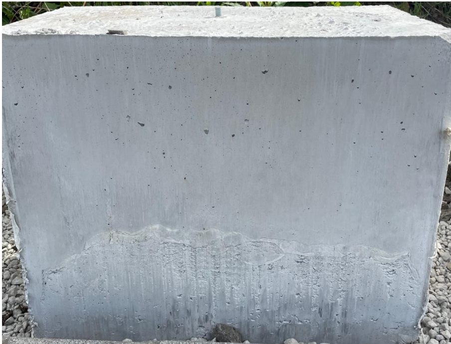
Figur 4.2-15. Betongoverflaten for 70BS.5SF.
